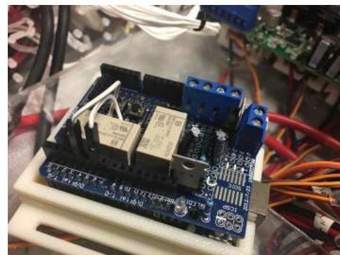
Fig 10. Lipo Battery monitor
