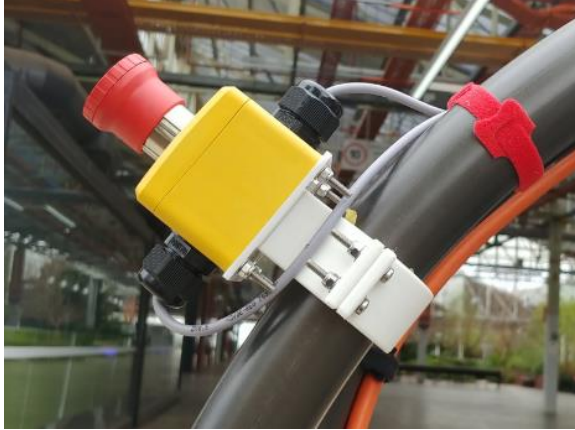
Figure 9: The redesigned e-stop mount, showing a three-piece modular design, this decision was made as it allows easy replacements of damaged parts.
