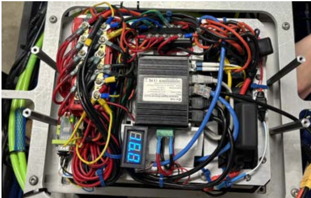
Fig. 42: New Electrical Stack – Populated, Top View
