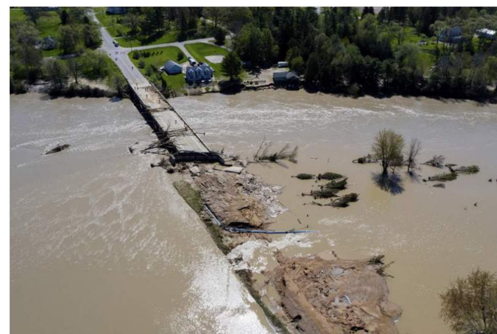
In this Wednesday, May 20, 2020, photo, people survey the flood damage to the Curtis Road Bridge in Ionia, Mich., over the Tittabawassee River. The bridge sits just south of Wilson Lake where the dams failed. (Neil Baker/The Grand Rapids Press via AP) (Neil Baker, MIWA)
